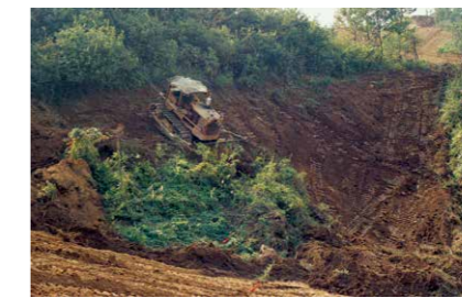
Circa 1969 Site preparation work underway Source: 17 juku no zosei koji (Site preparation of residential unit 17), Minamitama New Town Development Office document. From the collection of Tama City Cultural Foundation.
