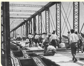
Just after the Great Kanto Earthquake. The army makes emergency repairs to the deck of the Azuma-bashi Bridge, which was destroyed by fire. Source: "The Reconstruction of Tokyo" published by the City of Tokyo.
